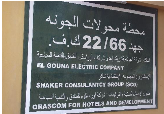
Figure 2: A sign of El Gouna Electric Company Station
