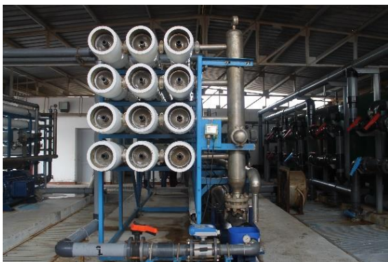
Figure 6: El Gouna Water Osmosis Station
