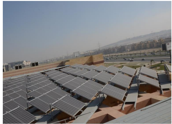
Figure 25: Solar Panels Installed over NUCA's Building (Farouh, 2016)
